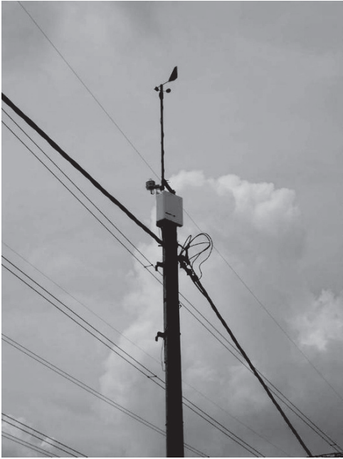
FIGURE 47.16 Weather monitoring using a weather station for transmission line in Malaysia.
